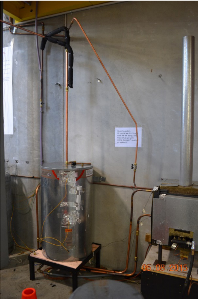
Figure 18. Cylinder below heater level. This test used a vent from the high point of the flow pipe connected to the cylinder vent, which allowed some circulation.
