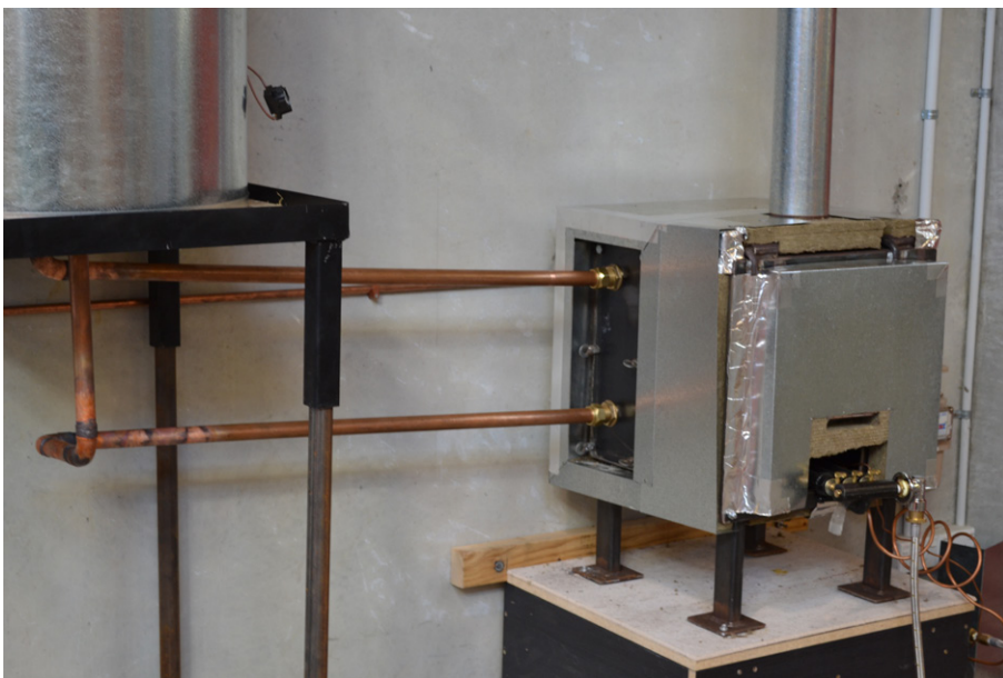
First test run, without lagging.
